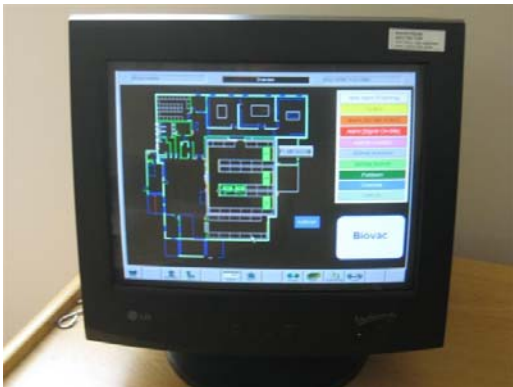
A2.9: Remote temperature monitoring
