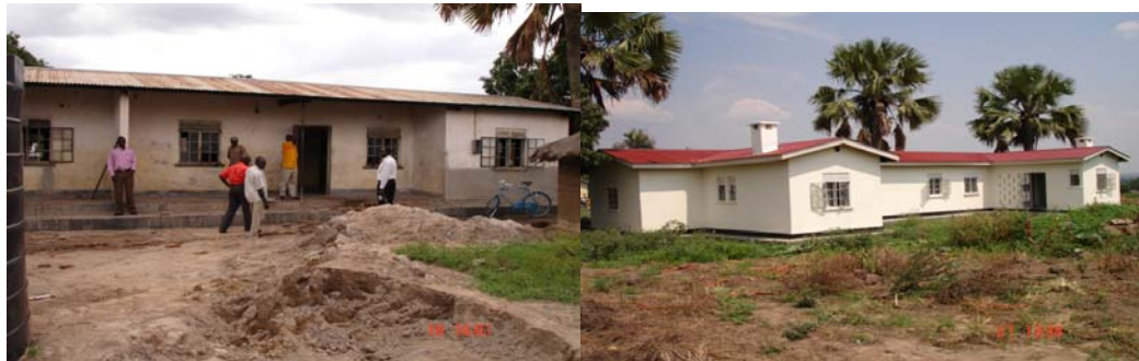
Amugo HC II staff quarter before renovation (front view) in March 2007 and after renovation (rear view) June 2007
