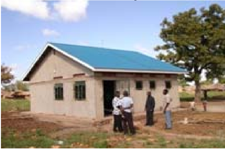
Figure VII: A WHO supported Maternity Ward under construction in Adwari sub-county, Lira District
