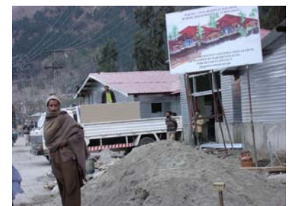
Ongoing construction works at the main hospital in Balakot. The construction is financed by private companies and individuals.
