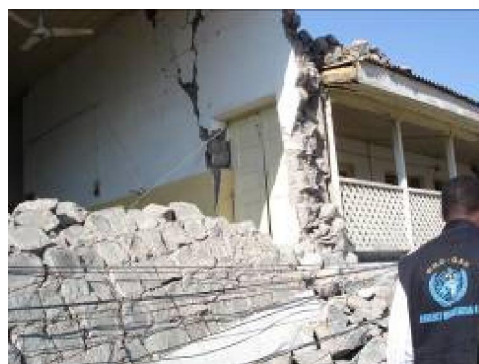
Earthquake damage at Rural Health Center- Abbaspur, Poonch, Kashmir, Pakistan
